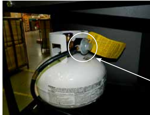
Gas connection @ tank
